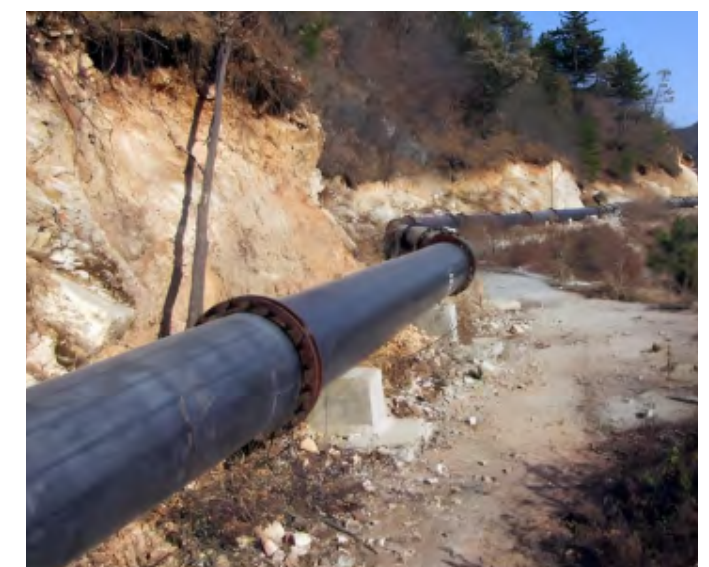
Mining Project, Slurry Transmission pipe
